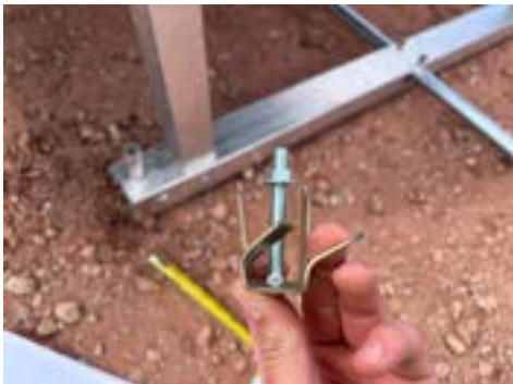
PHOTO 13: Bracket deformation after testing
