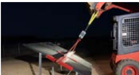
PHOTO 7: IR-30 Solar Racking System at max load
