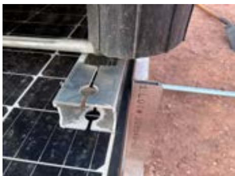
PHOTO 7: Slight deflections noted under load
