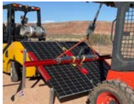
PHOTO 5: Test 1 - Evidence of ballast shift
